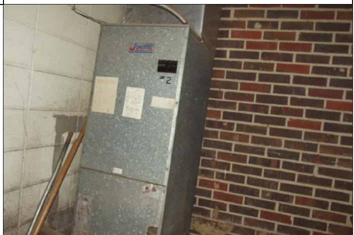
18. The Maintenance Office building has a split system which is abandoned-in-place.
