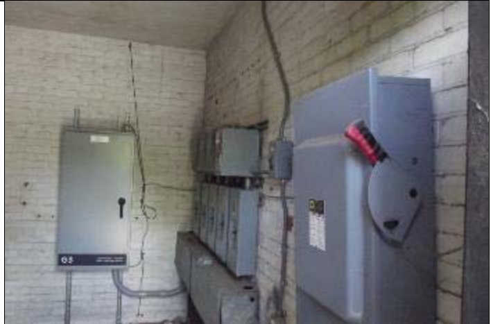
14. Main electrical switchgear in the electrical room.
