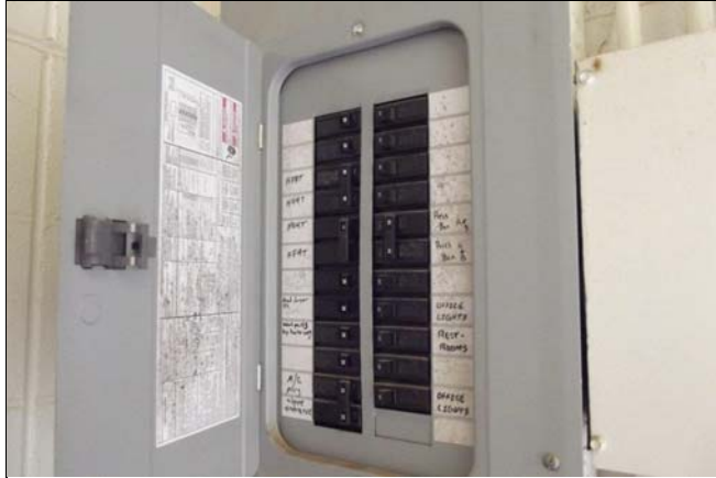
13. Typical electrical panel.
