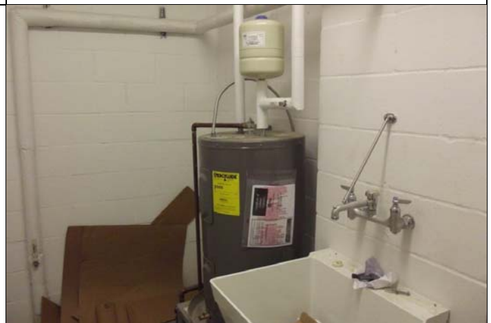
12. Domestic water heater in the Toilet Room building.
