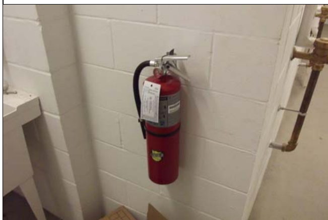
17. Fire protection is provided by portable fire extinguishers.
