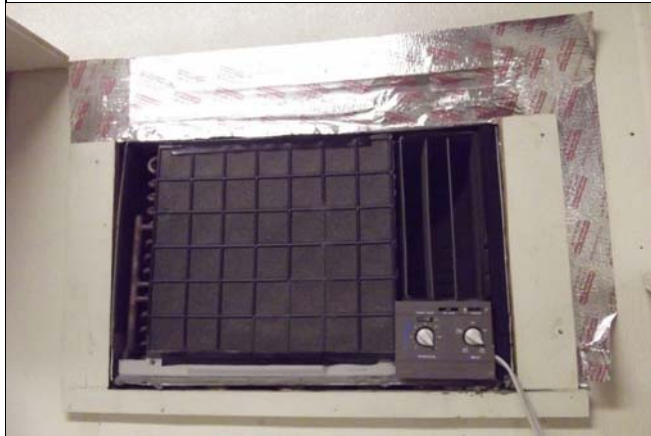
15. Heating and air conditioning is provided by through-wall package units.
