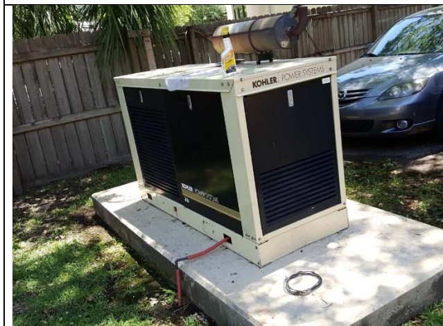
17. The Subject is provided with gas fired emergency generator.
