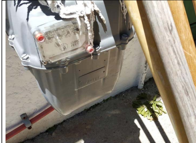
13. Incoming main gas service/meter is located at the southeast building corner.
