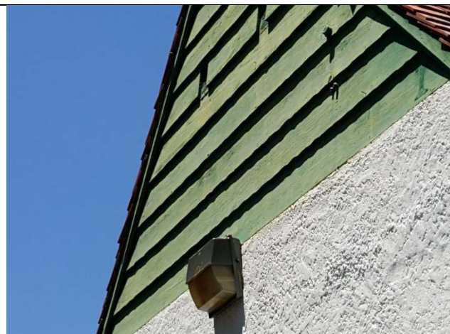
18. Site lighting is provided by building mounted fixtures.
