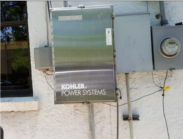
16. The main service panel disconnect switch, transfer switch, and meter are located on the east elevation.
