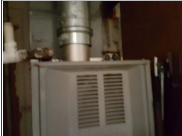
15. The AHU is located in a mechanical closet.
