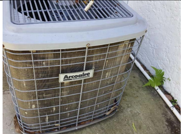
14. Air conditioning and heating is provided by a split-system with the condensers located outside the building.
