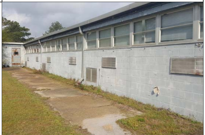
6. The original classroom building is a single story CMU bearing wall supporting steel structure.
