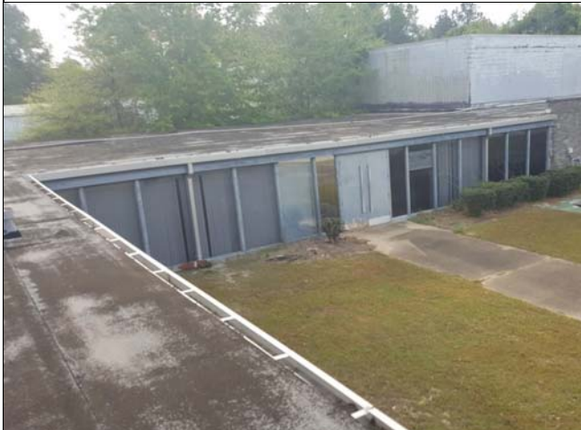
9. The roof over Classroom1 is a BUR that has perimeter downspouts and gutters.
