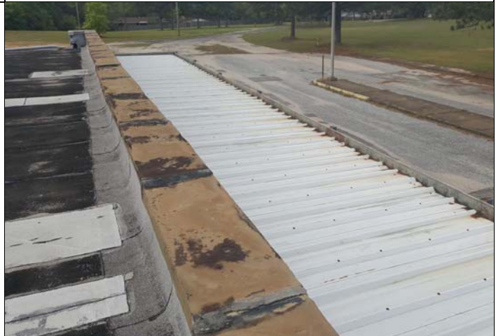
10. The parapet along the front of Classroom 1 has cast stone coping. The canopy is a metal roof structure.
