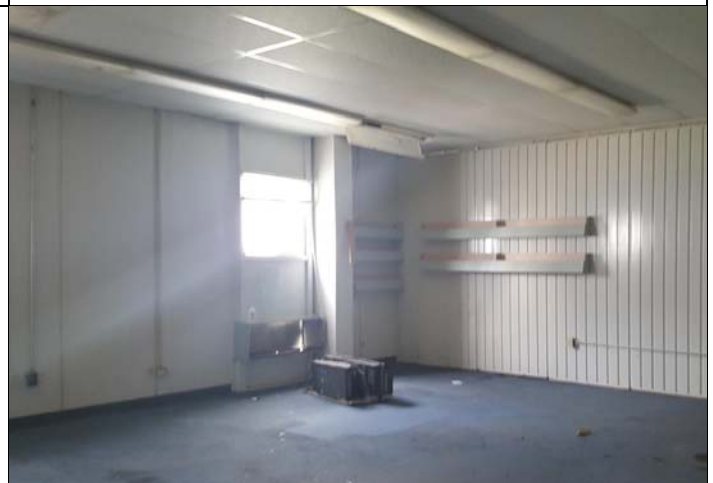
16. Classroom 2 is similar with double loaded corridors and classrooms on each side.
