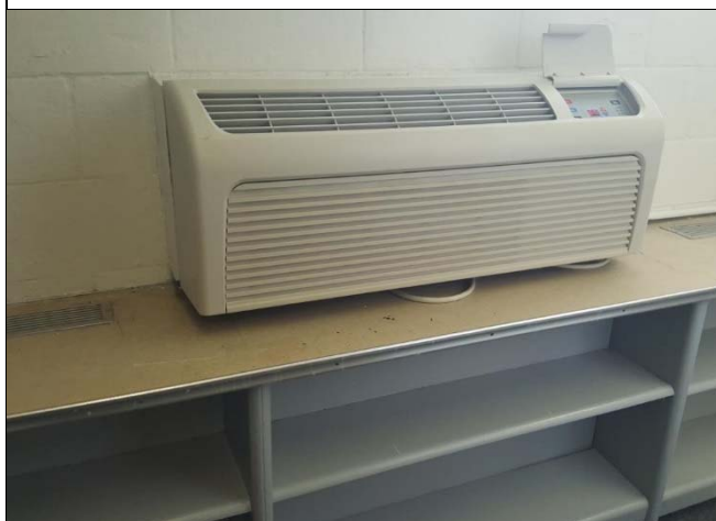
17. The central HVAC system is not used; some spaces utilize PTAC units.
