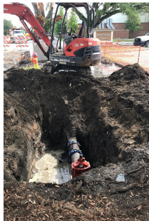
A new water line and valve are placed on the east side of N. Broad Street to St. Anthony Street.
