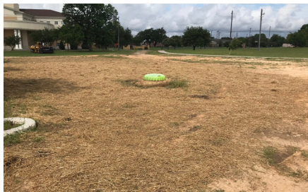
Crews placed fresh grass seed over the area where material and supplies have been stored to prevent sediment transport.
