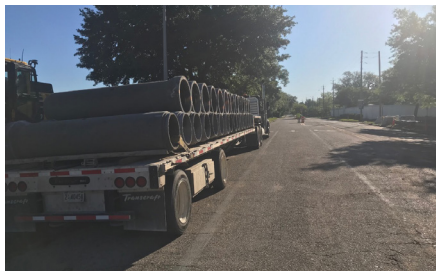
A truckload of reinforced concrete pipe for storm sewer construction is delivered to the project.
