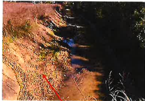
Slope and Bank Obstructions
