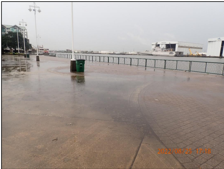
Photo 2 Areas of settlement behind timber bulkhead. Southern end of relieving platform, looking northeast.
