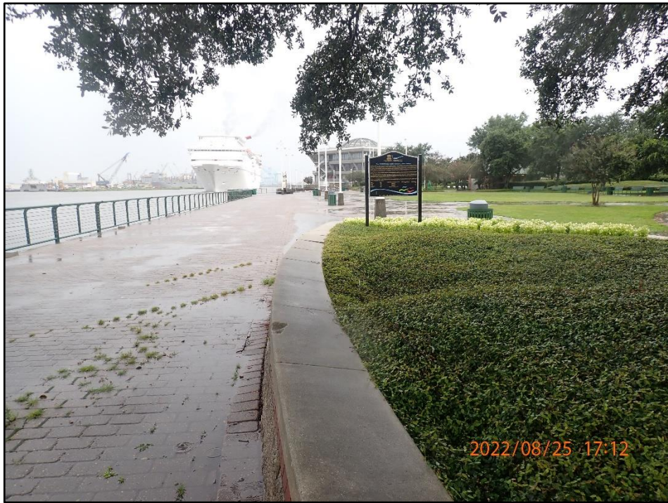
Photo 1 Planter wall rotation and areas of settlement. Northern end of relieving platform, looking south.
