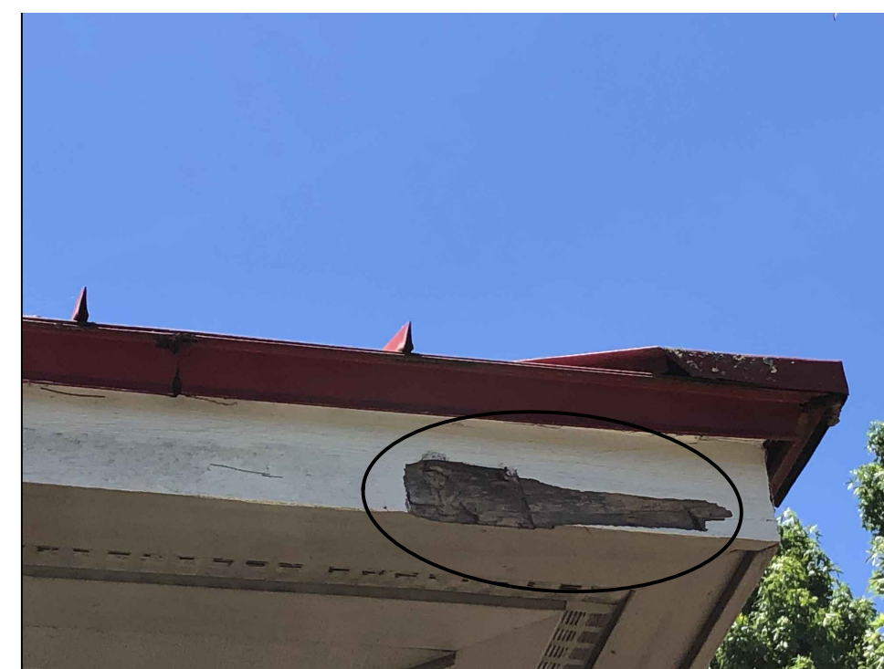
PAVILION PHOTO 06 • REPAIR/PATCH EXISTING FASCIA BOARD AT DAMAGED AREA.
