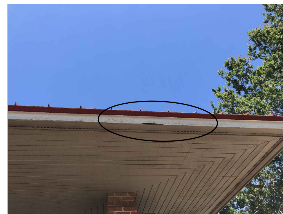
PAVILION PHOTO 07 • REMOVE AND REPLACE ROTTING FASCIA BOARD IN DAMAGED AREA.
