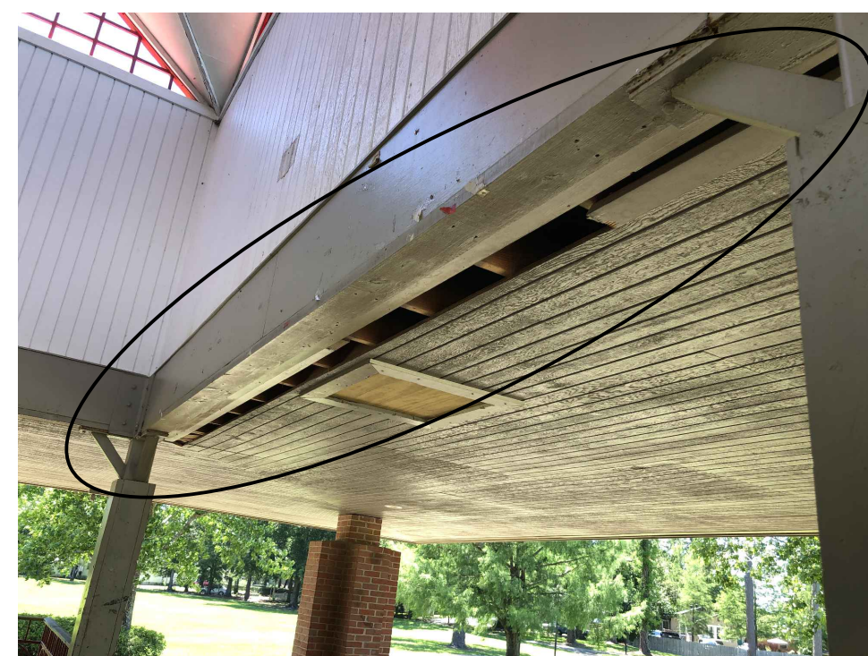
PAVILION PHOTO 05 • INSTALL NEW SOFFIT VENT AND NEW 1x TRIM TO MATCH EXISTING AT DAMAGED AREA.
