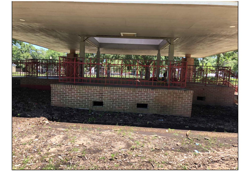
PAVILION PHOTO 02 • REMOVE EXISTING RAISED WOOD DECK PLATFORM WITH CMU, BRICK SUPPORT STRUCTURE & HANDRAILS. PREPARE FOR NEW CONCRETE SLAB
