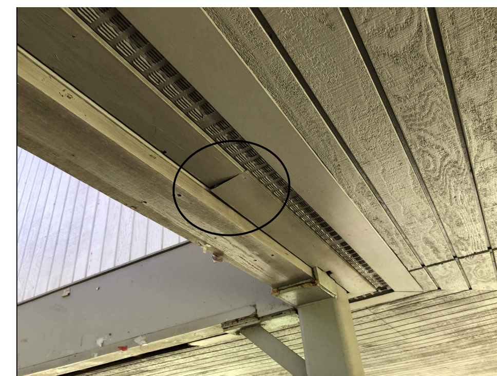
PAVILION PHOTO 08 • REFASTEN LOOSE TRIM BOARDS AS NEEDED.
