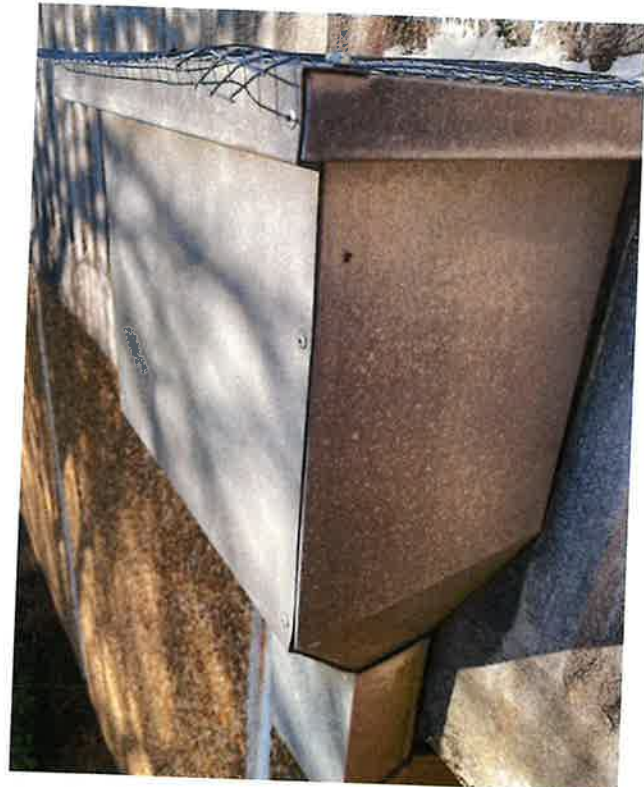
A leader head viewed from the side, with the downspout below.
