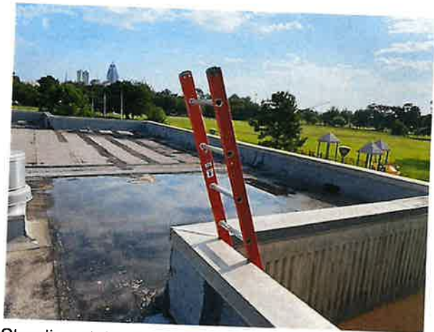
Standing at the east edge of the building, looking at Roofs 2 & 3. Roof 2 has standing water.
