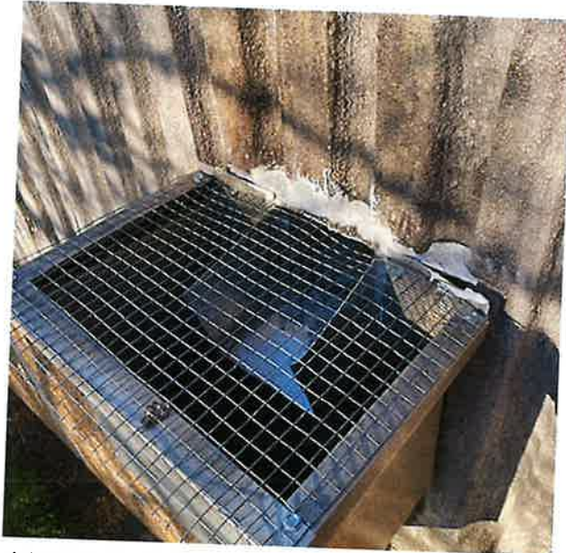
A leader head, viewed from above. The existing leader heads and downspouts are to remain.
