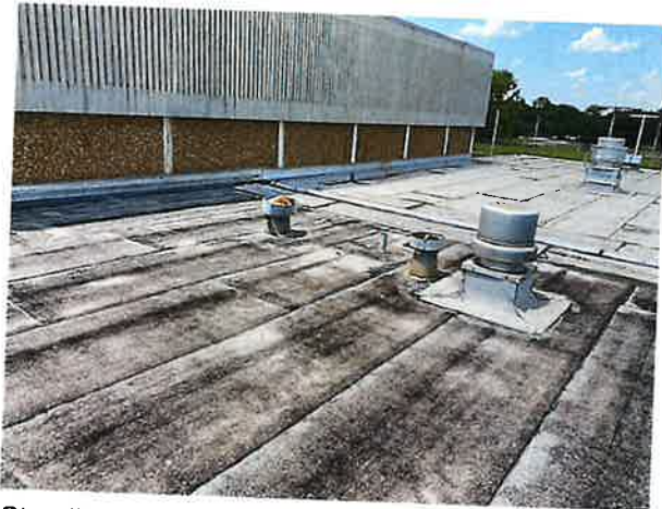
Standing on Roof 2 , looking across to Roof 3, with the gymnasium wall to the left.
