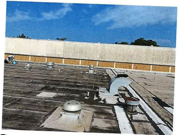
The east/west expansion joint that separates Roofs 2 & 3. The gymnasium wall is in the background.
