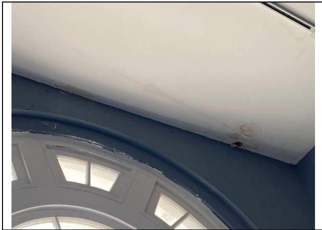
Photo #11. Water Damage Observed on the First SVMG Floor Ceiling
