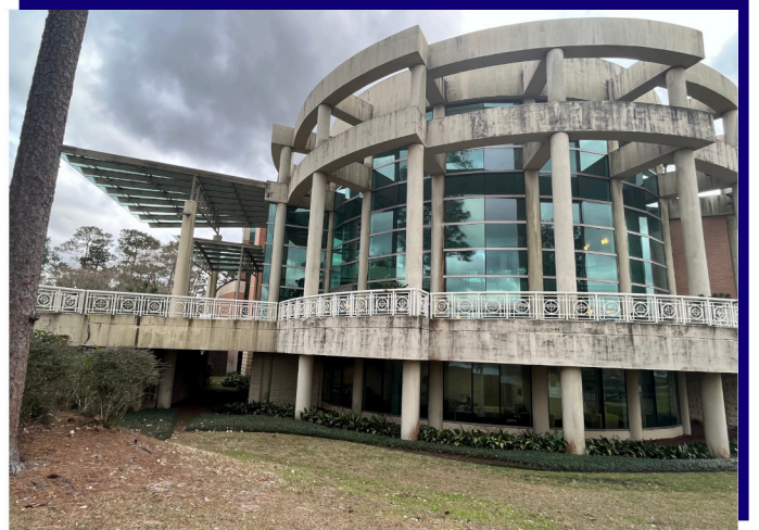
Window wall at entrance requiring gaskets to be replaced
