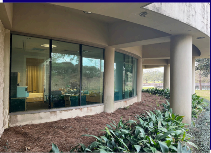
Office windows below entrance requiring gaskets to be replaced
