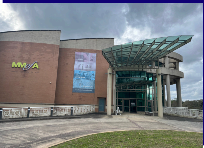
Window wall at entrance requiring gaskets to be replaced
