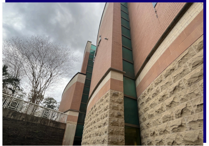
Vertical window strips left of the entrance requiring gaskets to be replaced
