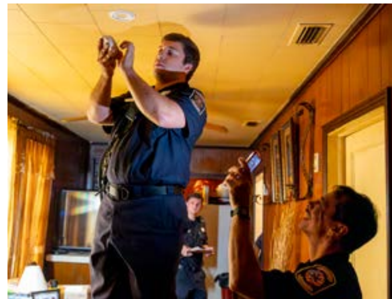
October 9 Homes in the Plateau community get free smoke alarms installed during a smoke alarm blitz.
