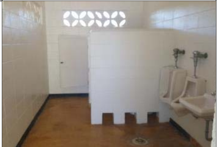
10. Two multi-user toilet rooms are accessed from the exterior to support the ball fields.
