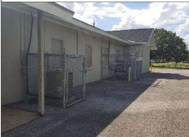
5. The east elevation has two condensers enclosed by chain link fencing.
