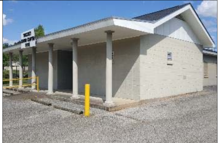
2. The exterior wall is painted CMU, which is a bearing wall supporting the wood structure.
