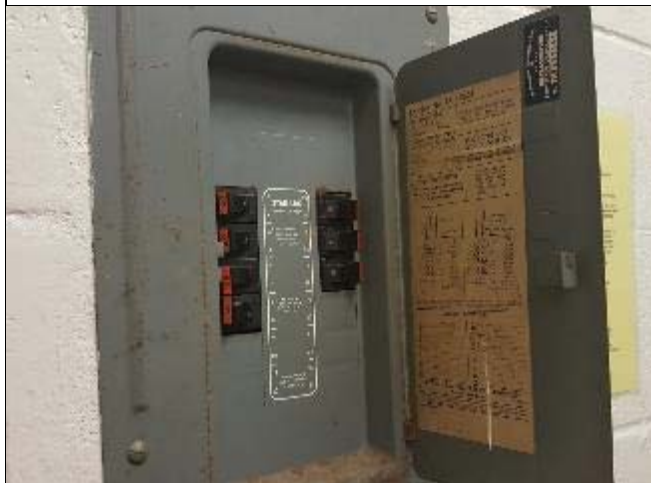
15. Stab Lok distribution panels were observed.
