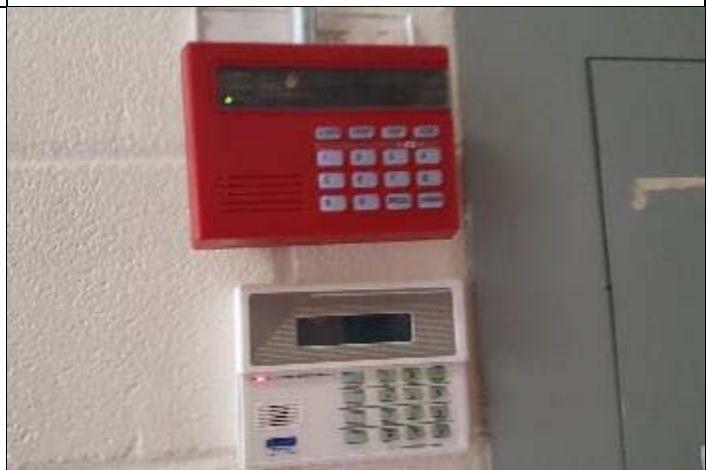
18. A fire alarm and security panel are provided at the front of the facility.
