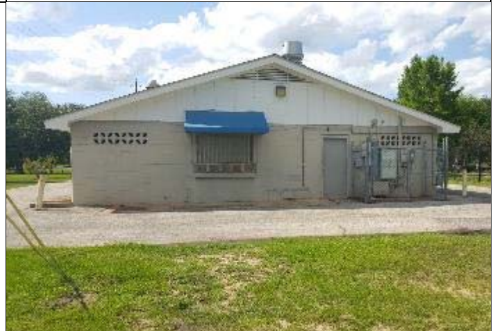
4. The rear elevation of the building has a window with a fabric awning and the electrical service.
