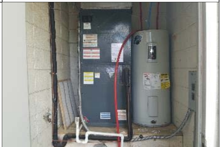
12. The building is heated and cooled by split systems and DWHs provide hot water.
