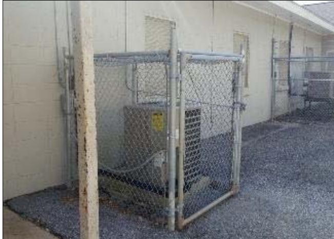
13. Split systems are located at grade in chain link fence enclosures.
