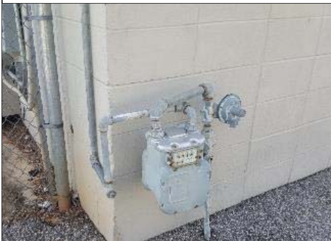
11. A gas meter is located at the southeast corner of the building.
