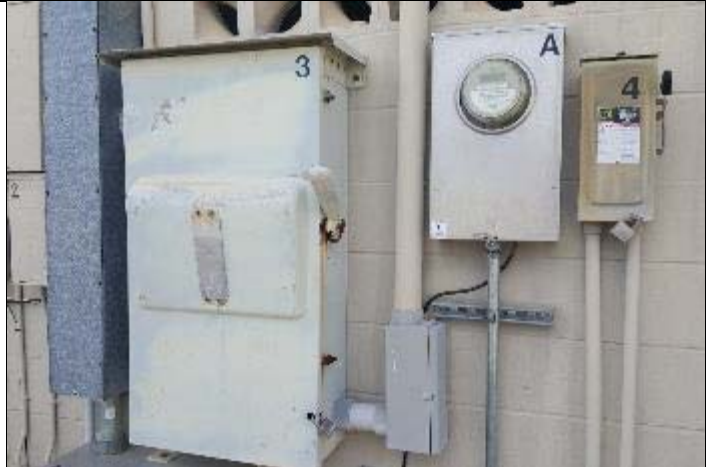
14. The main electrical service enters the Subject into the south side of the building.
