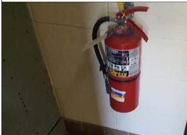
17. A wall mounted fire extinguishers is located at the front vestibule.
