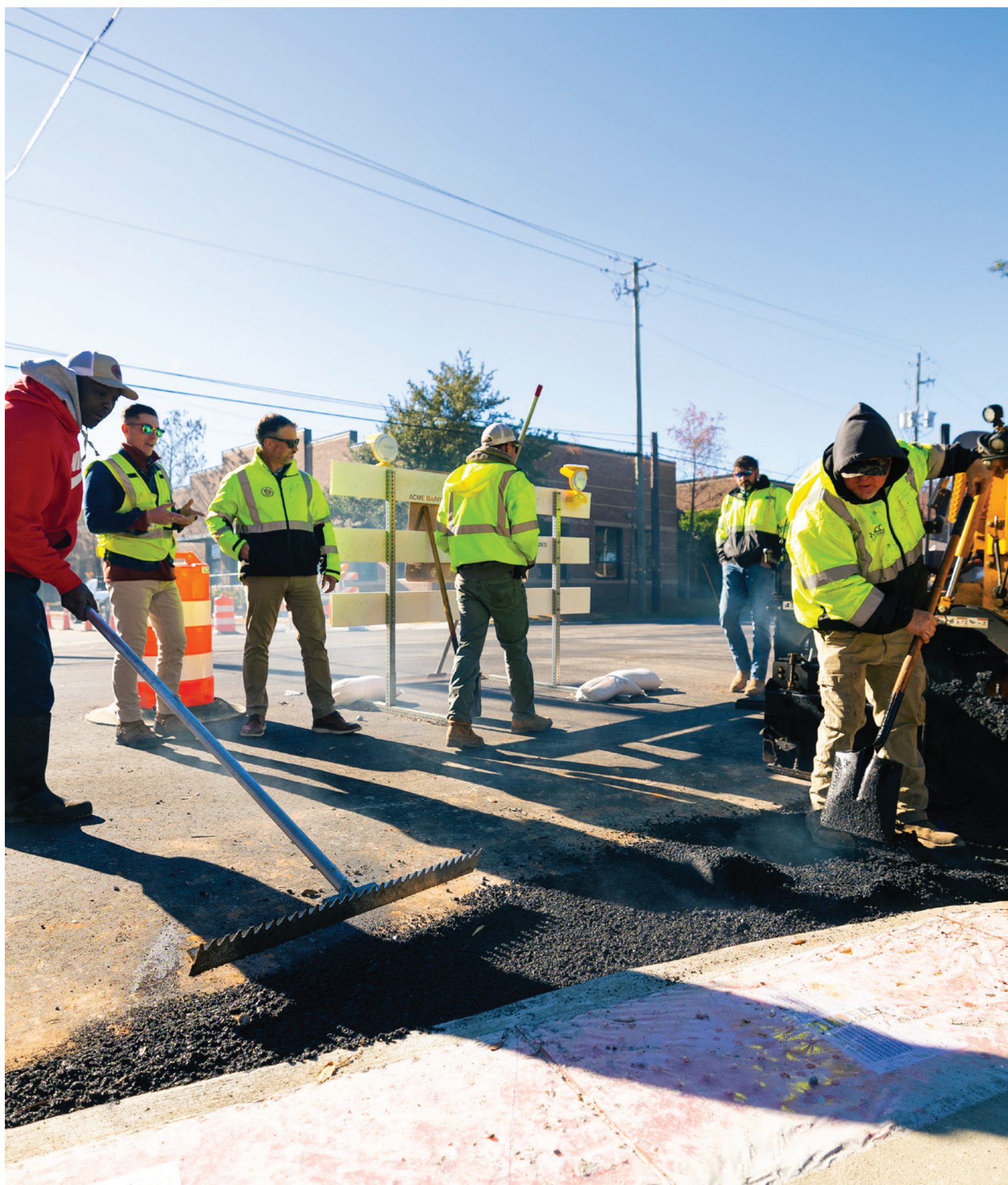
Members of the Capital Engineering team oversee the successful completion of the North Washington Avenue culvert repair as the final layer of asphalt is laid.
