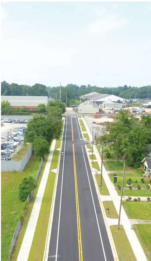
The newly renovated Ann Street project features culvert replacement, curb and gutter repair, new bike lanes, and fresh sidewalks.
