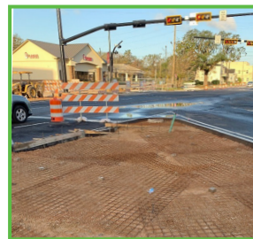
Crews finish up the slope paved nose. This is the sloped concrete seen at the end of a median or island.
