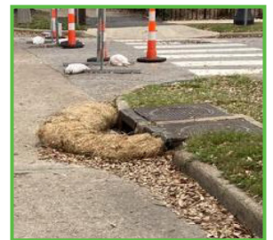
Crews are working to replace any aging or damaged erosion control devices.
