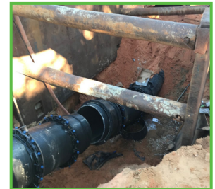
Crews working on the sewer system are tying in a waterline bore stub.
