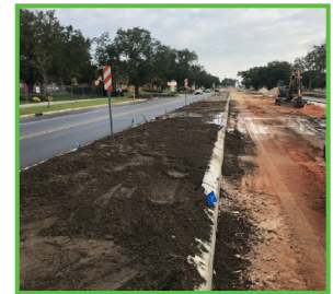
Crews add topsoil to a newly constructed median after installing the irrigation system.
