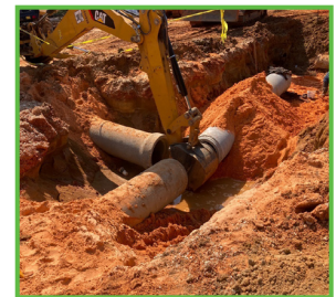
Crews place new storm sewer lines in the proper alignment for a new junction box.
