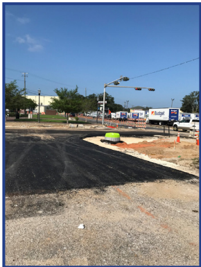
Crews created access to a business on North Broad Street near the St. Anthony Street.
