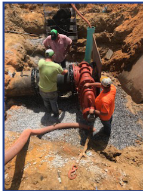
A new 24-inch water valve is installed below the roadway at Springhill Avenue.
