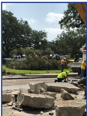
Demolition of existing roadway at South Broad and Canal Streets is underway.
